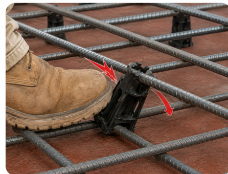
Accidental contact during construction
